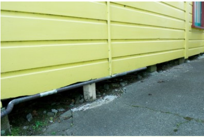
Figure 7: Areas of subfloor space with insufficient clearance
