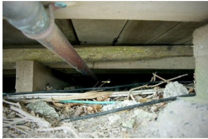
Figure 8: Areas of subfloor space with insufficient clearance
